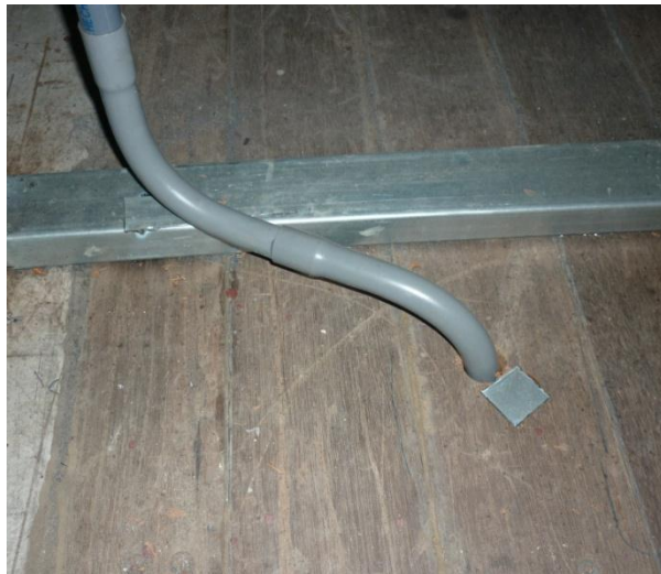
Conduit pipe passing through hole in the floor
